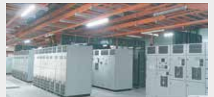
Successful integration with the LV electrical system
