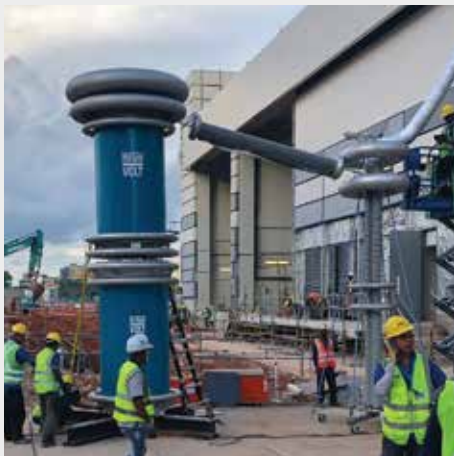
230kV GIS Equipment Testing
