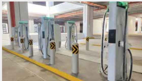
LTA EV Bus Depots (Sengkang West & East Coast)
