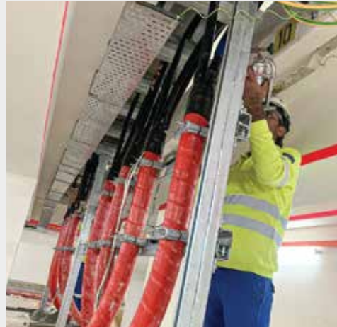
HV cable at the substation cable chamber room, ensuring the proper functioning of the high voltage cabling system
