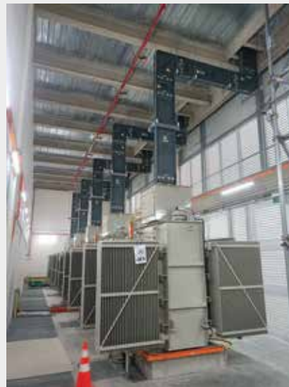
Supply and installation of LV busduct between the transformer and the main switchboard
