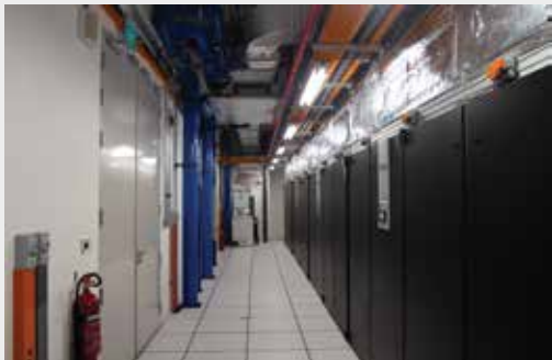
Computer Room Air Conditioning (CRAC) Room
