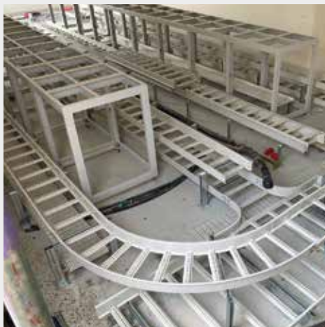
Our team successfully installed cable ladders as supports for high-volume or heavy cabling
