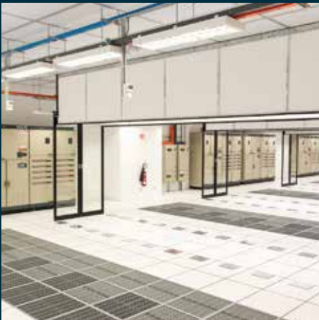
Hot Aisle Containment with raised flooring, dual sliding doors, and vinyl Rack Hat between the ceiling and cabinets.
