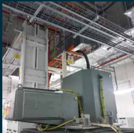
Electrical Power Distribution Network & Cabling Works - Indoor busducts & termination work to transformer, cable containment & cabling works
