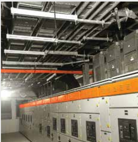
Busduct connection to switchboard
