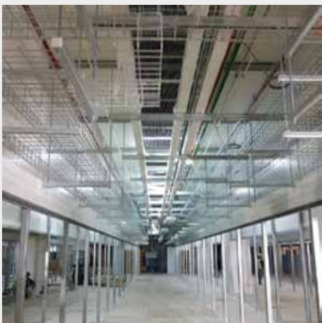
Customised metal fabrication works - customised cable support system in hot aisle for future M&E services installation
