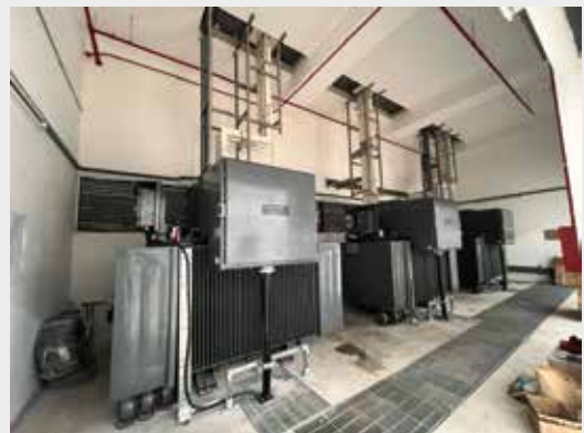
2.5 MVA FR3 Oil-Type Transformer (51 Benoi Road): Full supply, installation, and commissioning. System energized and handed over ahead of schedule.
