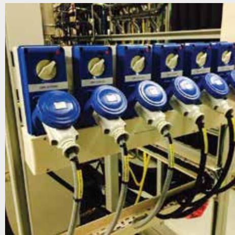
Supply & Install LV Provision of industry socket (Ceeform) for hook-up of wafer-chips Fabrication
