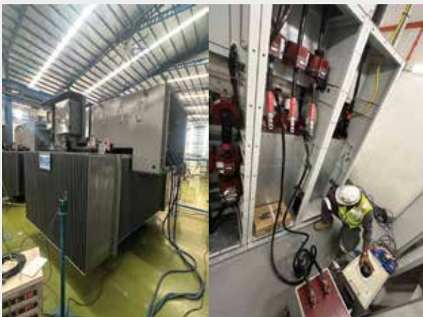
Testing & Commissioning: Rigorous FAT and SAT conducted to ensure all equipment met safety standards and was ready for site deployment.
