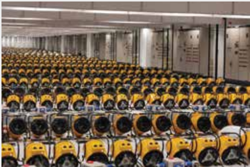
4 Mega Watt Heat Load Test (4MW HLT) during Integrated System Test (IST)
