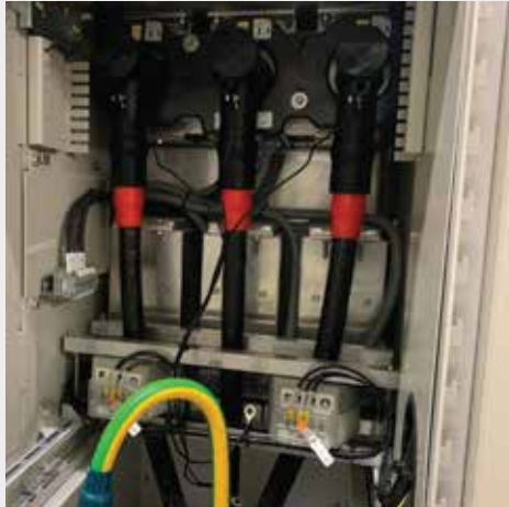
Completion of termination work for 22kV at the switchgear was a critical milestone in the project
