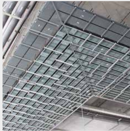
Securely mounting busducts to unistrut supports and aligning ends of adjoining sections.
