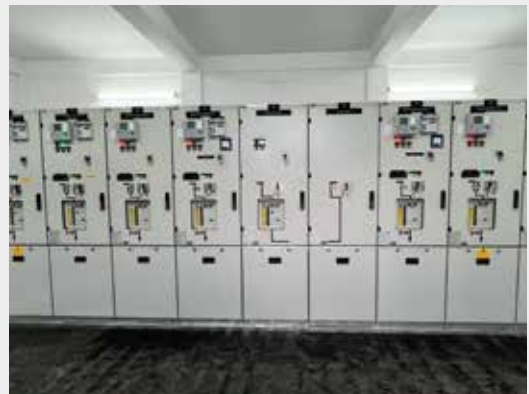
HT Switchgear GIS ZX0 (2A Mandai): Full supply, installation, and commissioning. System energized and handed over ahead of schedule.
