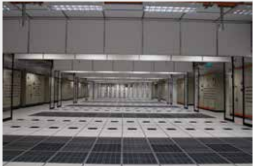
Hot Aisle Containment setup
