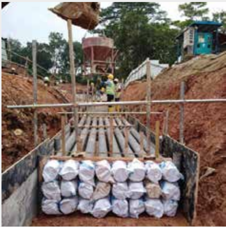
Underground Electrical & telecom Lead-in Pipe works: Concrete haunching of pipes in progress
