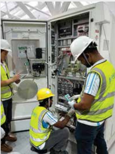
Testing and Commissioning of 120kW DC Charger
