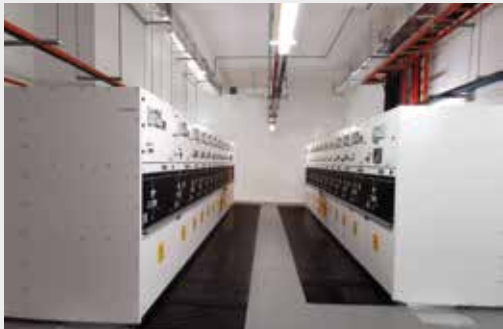
High Voltage (HV) Switchroom
