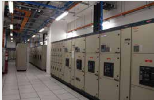
Low Voltage (LV) Switchroom
