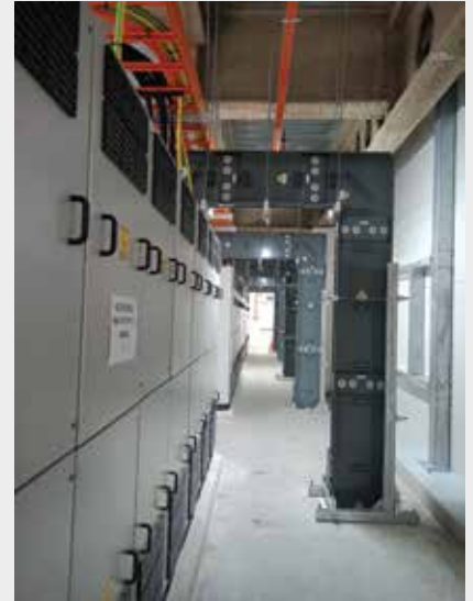
The busduct riser facilitates vertical power distribution across the building's floors
