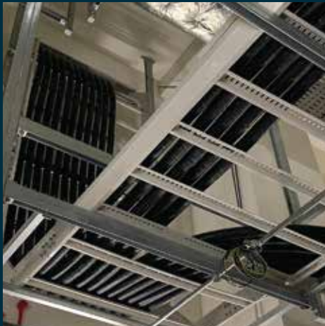
Successful installation of the HV 12.7/22kV cable on the cable ladder system
