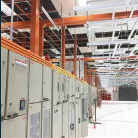
BMS / EBMS Installation
