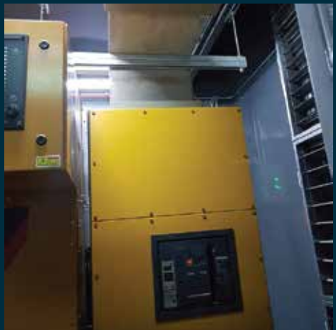
Electrical Power Distribution Network & Cabling Works - Cast resin busducts & termination work inside generator enclosure
